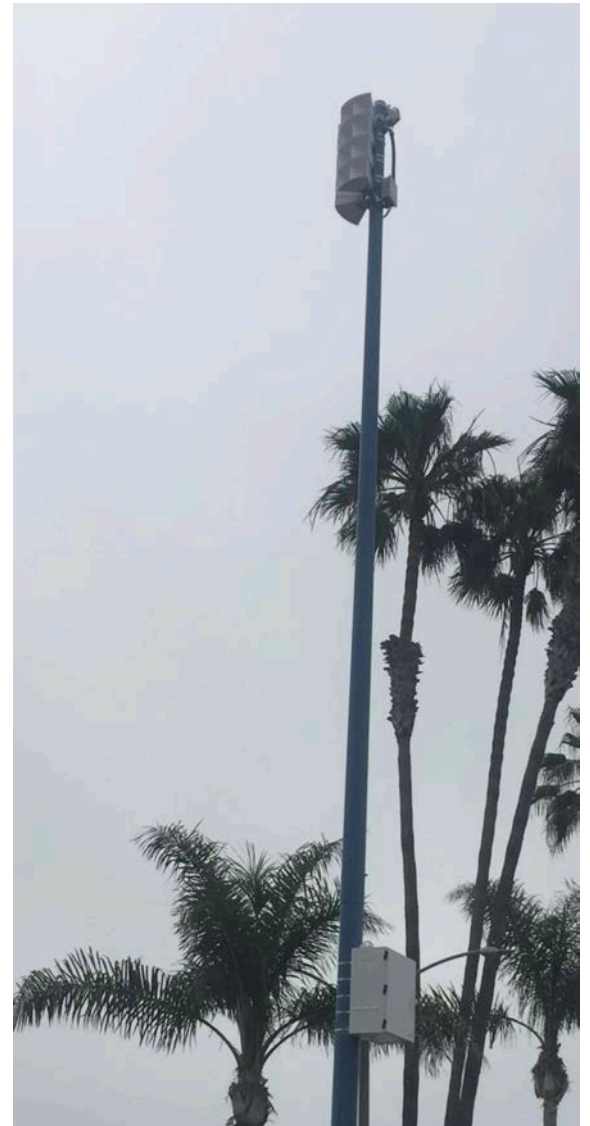
GENASYS VOICE SIREN - WEST JETTY PARK INSTALLATION
